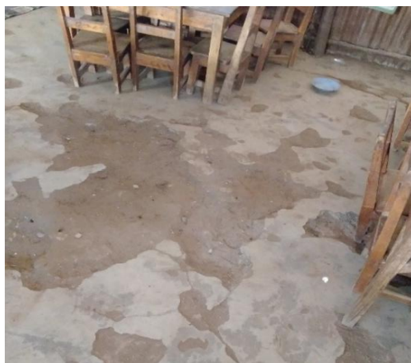
Figure two: Rough, uneven cement floor in a pre-school classroom in Mombasa
